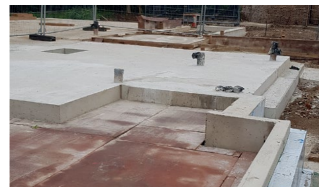
NEW FOUNDATIONS The concrete slab for the café, kitchen, toilets and staircase
